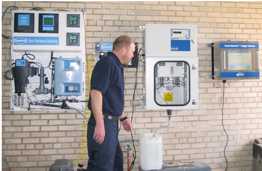
Fig. 2. A real world deployment site showing the system in operation.
