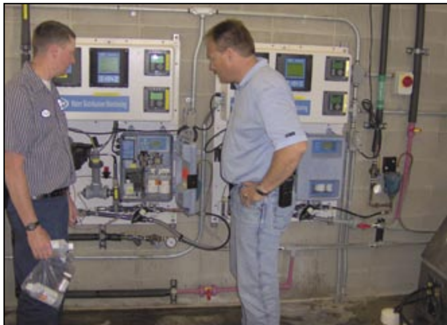
Wastewater Lab Manager Dennis Spilman (left) and Superintendent Kevin Moler inspect the Hach Water Distribution Monitoring Panels at the Clear Lake (Iowa) Sanitary District. Operators typically clean the sensors and check split samples against portable meters once a week.
